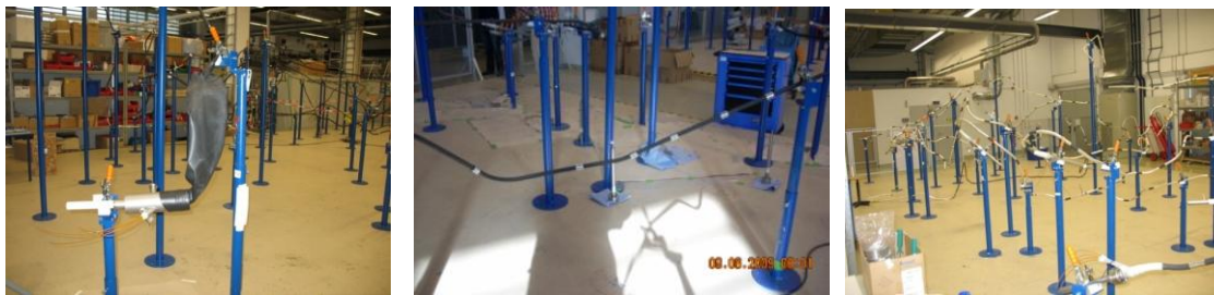
Fig.13 A bus bar end during Paschen test (left), Al sleeves glued (centre), bus bars covered with thermal insulation (right)
