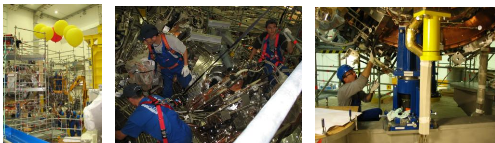
Fig.14 Final installation of the bus bars on module 1: transportation of the bus bars to module 1 (left), fastening of the bus bars in holders on top and bottom of the module (centre and right)
