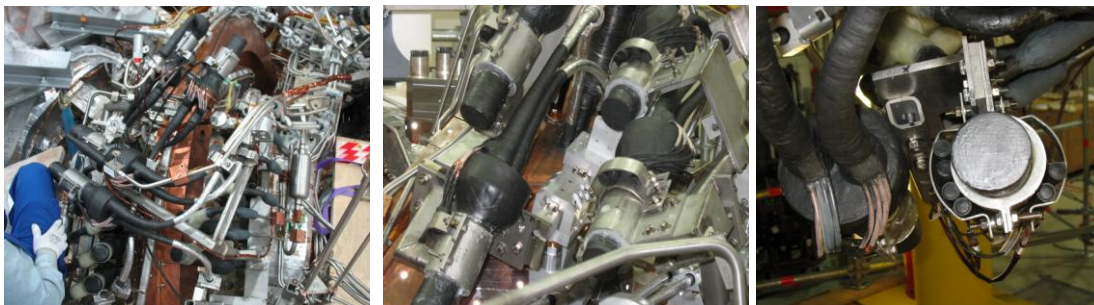
Fig.21 Joints equipped with QD system, painted with black conductive lack and clamped to coil structures
