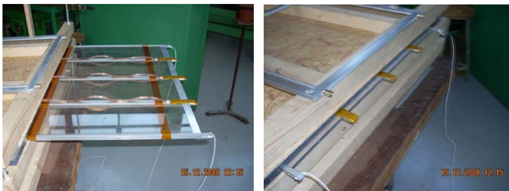
Fig.16 Dummy module inserted by hand to the outermost tower; two cables tightened to the top and bottom C-profiles to be used to pull the module out
