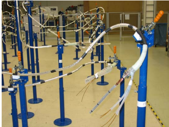
Fig4. Bus bars ready for the final installation
