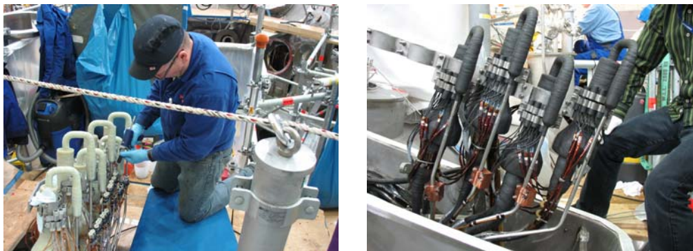
Fig.13 Casting of QD boxes (left); finished QD system of non planar coils (right)
