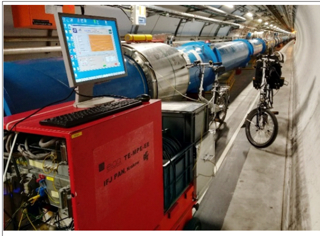
Fig. 8.5b. Standard ELQA measurements in the LHC during Long Shutdown 2. (Image copyright DAI).
