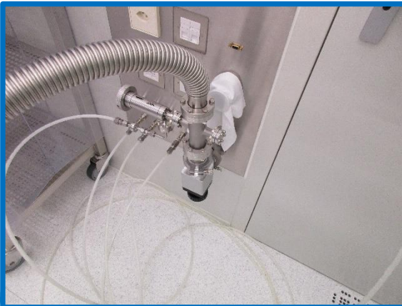
Panel inside cleanroom
