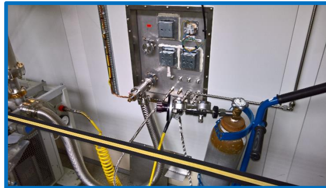
Panel outside cleanroom
